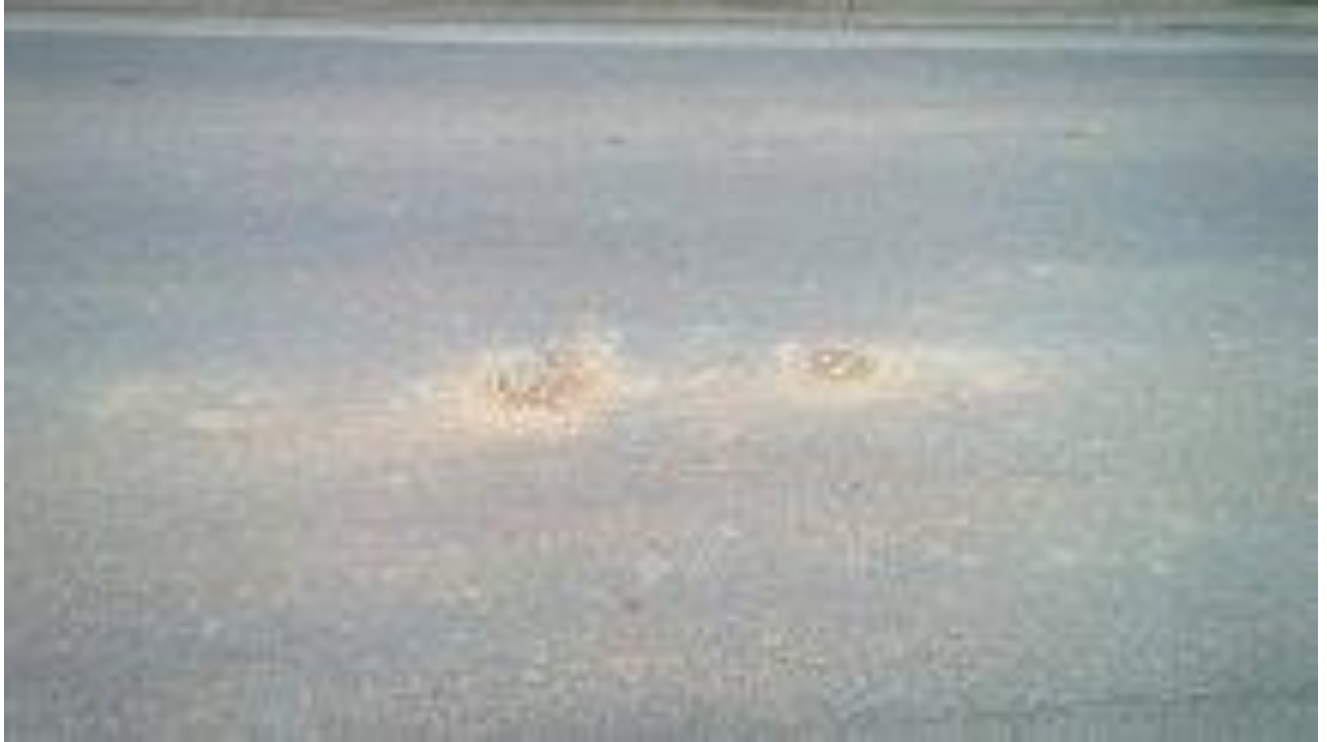
Globs of mud and gravel adhering to WP Rd. even after sweeping
