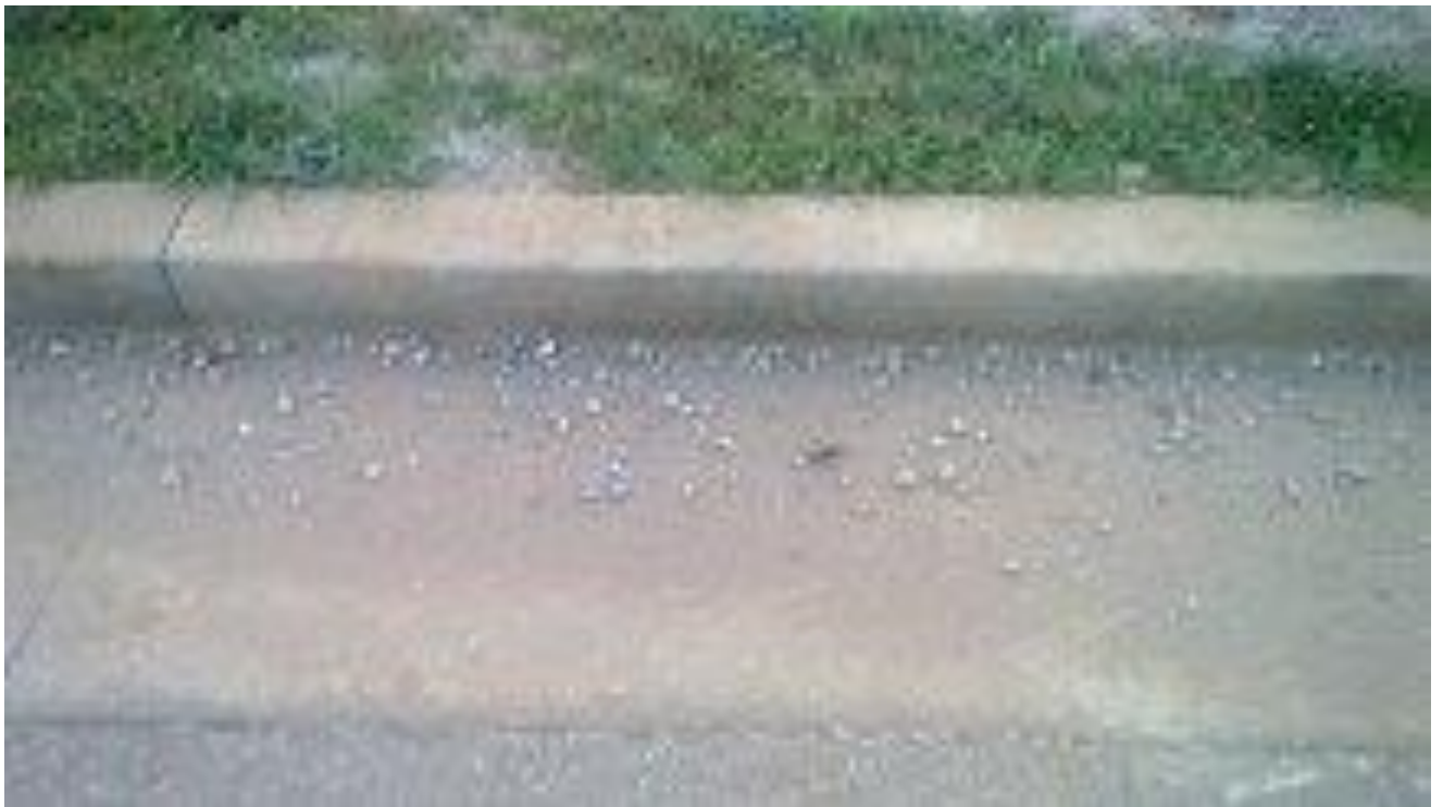
Gravel along curb on WP Rd..
